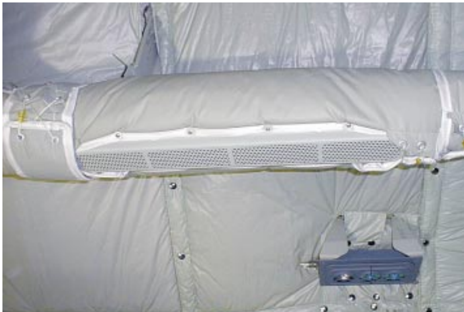
Old style cargo compartment heating duct - air is directed straight down onto window when door is open and locked in overhead position.
