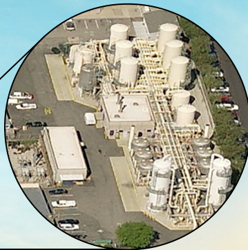
Burbank Operable Unit Treatment System
