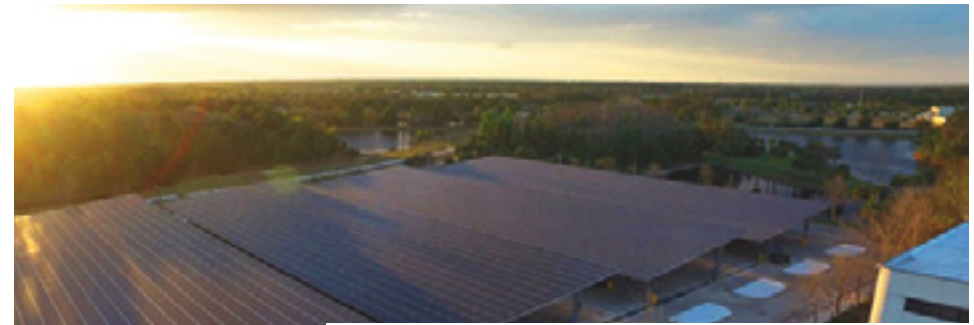
Solar Carport in Orlando, Florida.
