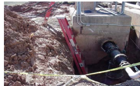
Not properly sloped, benched, etc.
