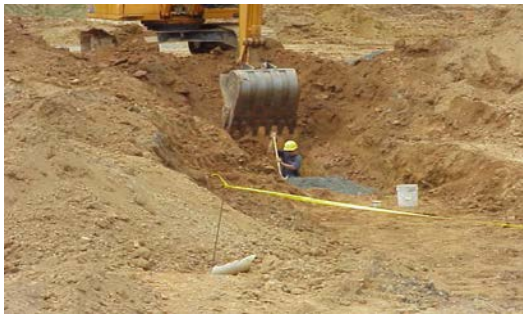
Not properly sloped, benched, etc.
