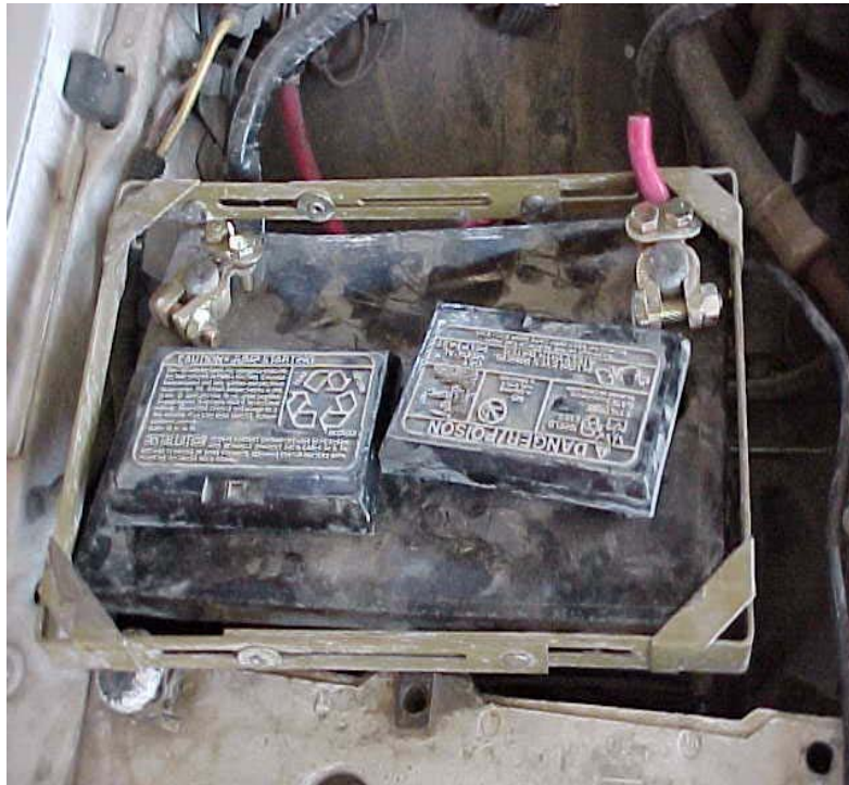
Top Cover Loose / Not Wired
